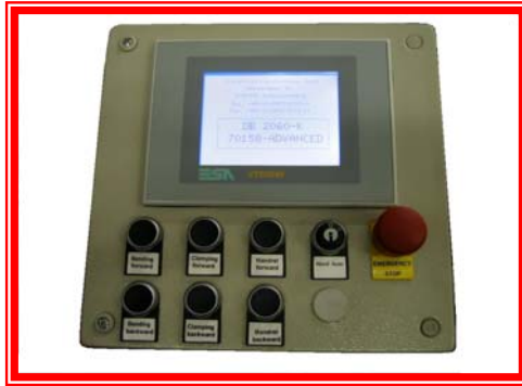
SPS control panel
